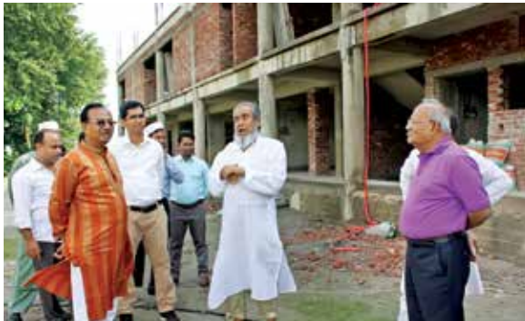
Al-Haj Nur Mohammed, Chairman, Jamuna Bank Foundation alongwith Mr. Kanutosh Majumder, Chairman, Jamuna Bank Limited visited the construction site recently to monitor the construction works of the "Old home".
